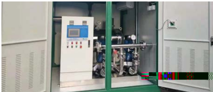
Temporary Water Supply
